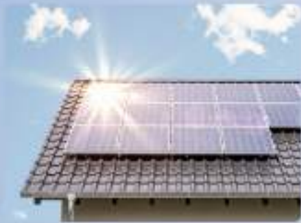
Solar Panel System with Battery
